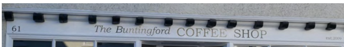
Figure 24 - Various sign and fascia issues
