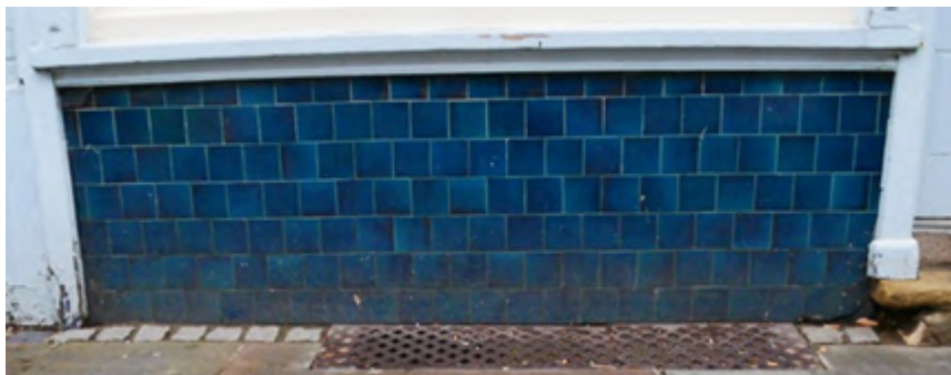
Figure 30 - Glazed blue tiles appropriate to this stallriser.
